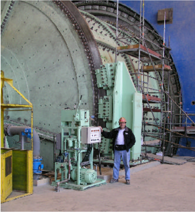
Twiflex 6 Caliper Mill Braking System installed on a Metso 40' SAG Mill at Collahuasi Copper Mine in Chile.
