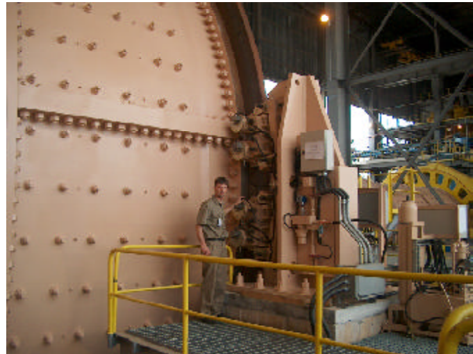
Twiflex 4 Caliper Mill Braking System installed on a Metso 38' SAG Mill at CVRD's Sossego Copper Mine in Brazil.
